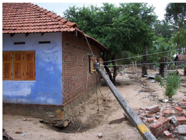
圖 2，斯里蘭卡沿岸房屋周圍土壤受海嘯淘刷痕跡。出處 ( http://coastal.usc.edu/plynett/Sri%20Lanka%20Tsunami%20Damage/slides/d2_scur5.html )
