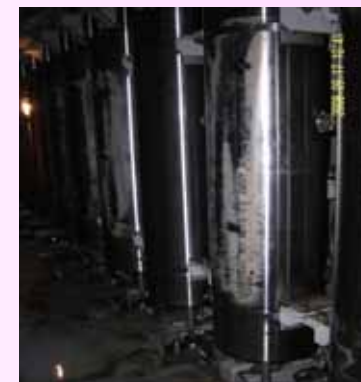
#1RB EL-8200 CRD HCU Room
